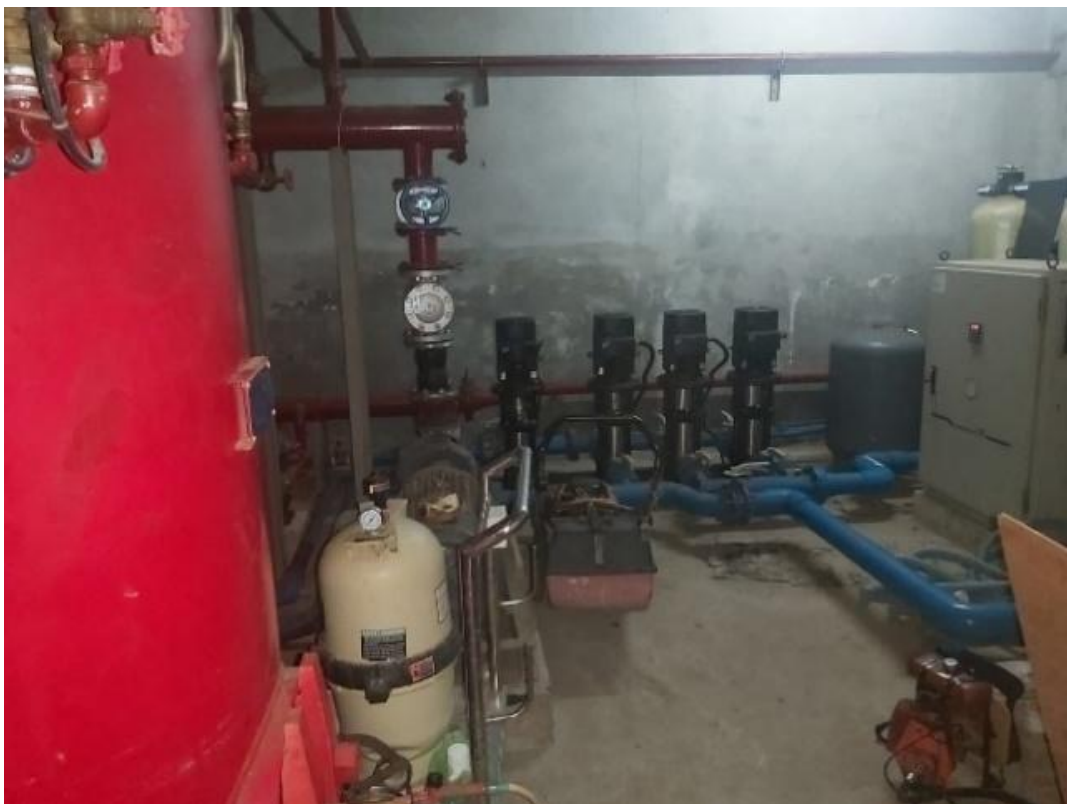
Figure 3. Water Treatment for Water Efficiency in Hotels [Source: Research Documentation, 2025]
